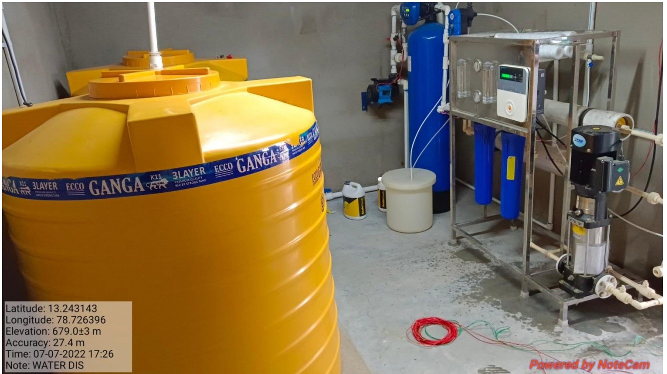
WATER RECYCLING SYSTEM
