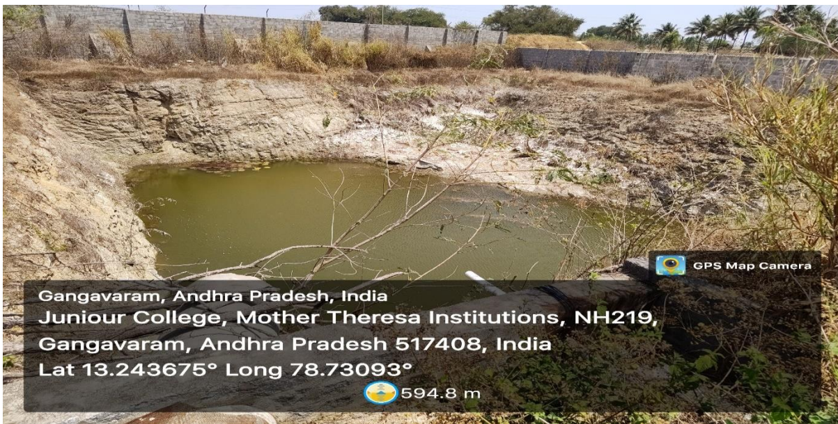
PERCOLATION POND CONSTRUCTED TO COLLECT RAINWATER AND FOR WATER RECHARGE AT FIELD
